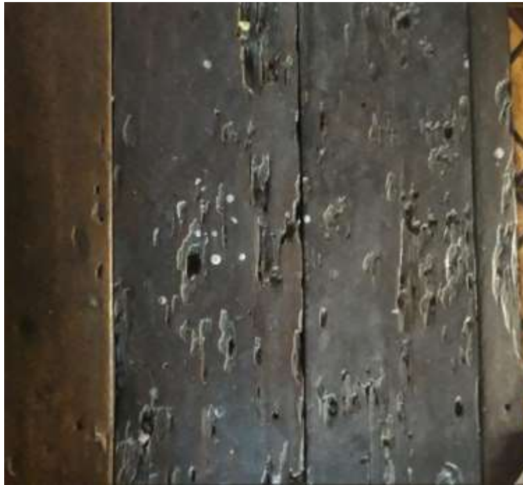
Photo 20. The condition of the floor in an old building that has been eaten by termites (Photo: Ismuha Nurul Hayati)
