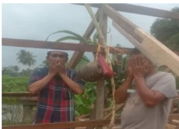
Figure 1. Installation of naek bukkulan attributes in the form of plants when raising the house rabung before being given a roof.
