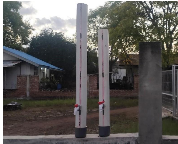
Figure 4. Rapid Sand Filter (RSF) Filtration Unit
